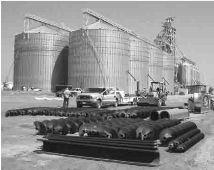
Typical installation of screw conveyors at a large grain storage facility.
